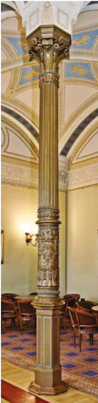
11a. Iron column in the former Library of the Academy (photo Hámori, Péter, 2017)
