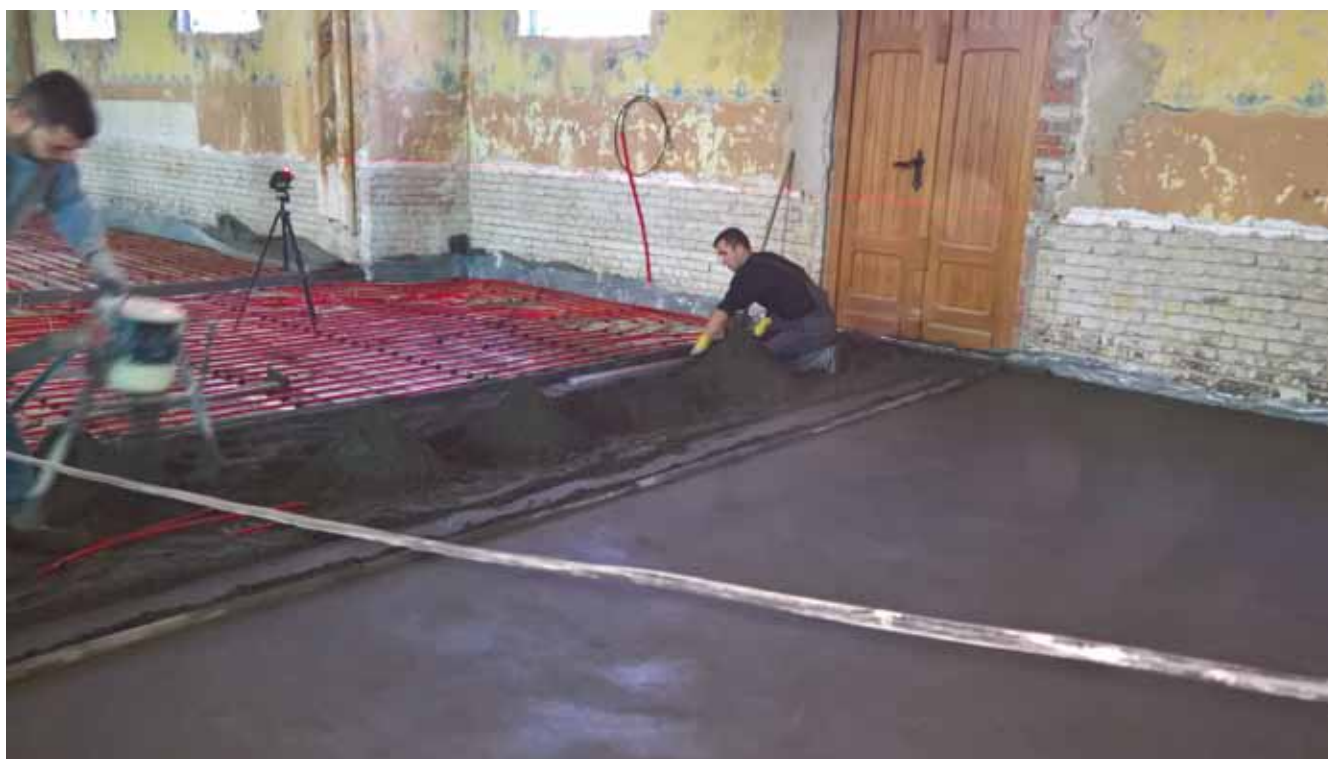
5. Under-floor heating through a system of pipes
