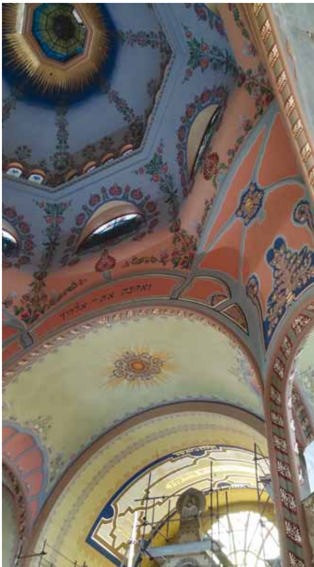
8. Secco tempera wall decoration (The plaster shell under the dome is about 7–8 cm thick)
