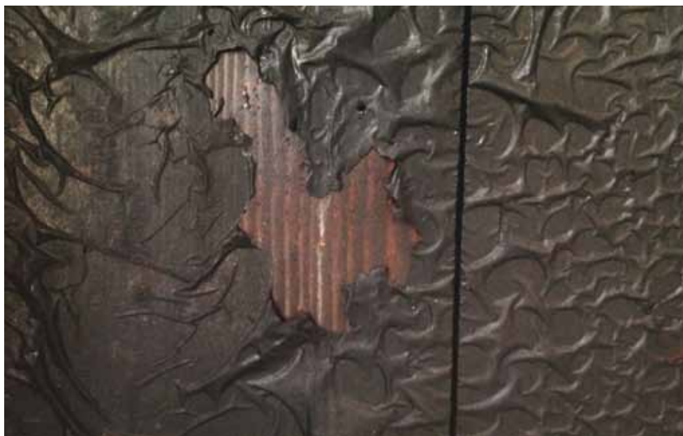
5. Blistered timber panel, first floor corridor, Mackintosh Building, May 2014
