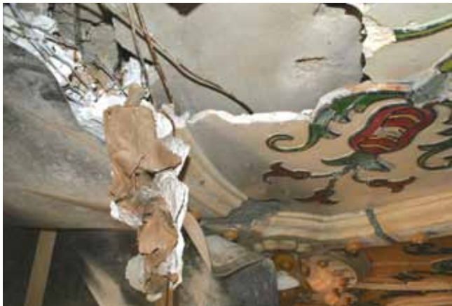
10. After the cleaning and the removal of the ceiling ceramics in bad condition, the problems turned out to be critical
