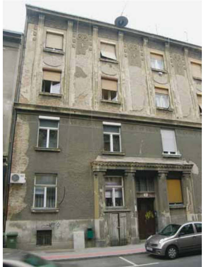
9. 80 Palmotićeva Street: Façade before the restoration
