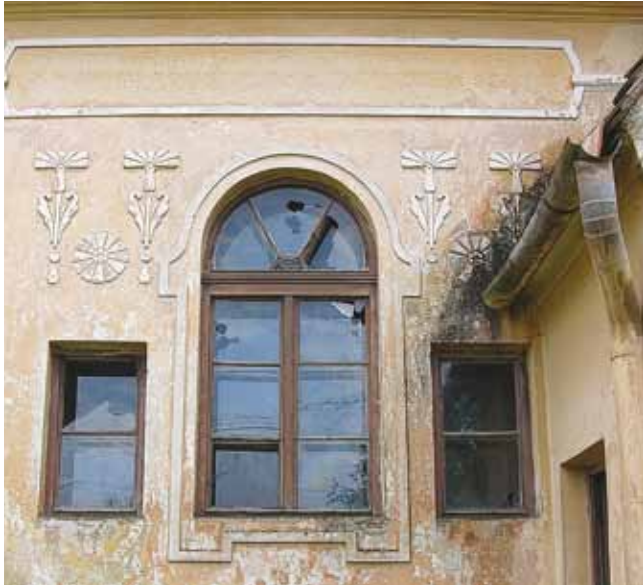
9. Former Lutheran School in Cincșor in 2008, detail of deteriorations
