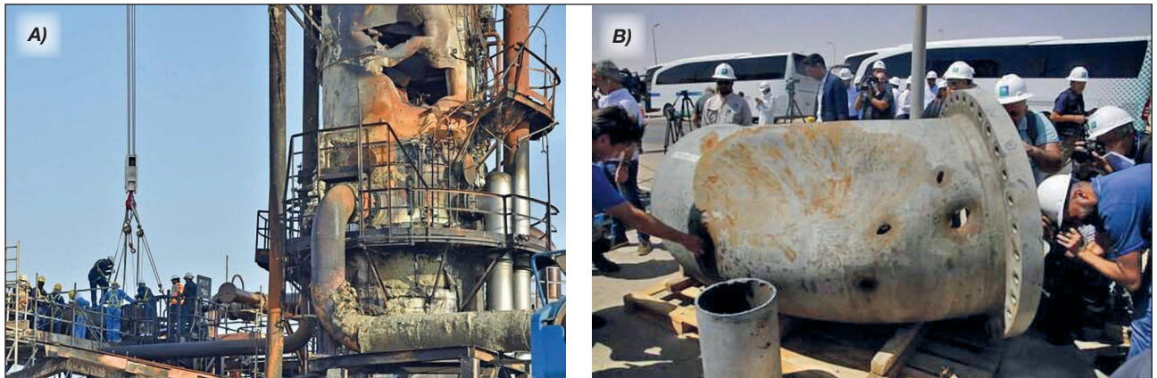
Figure 2. Closer look at the damages
