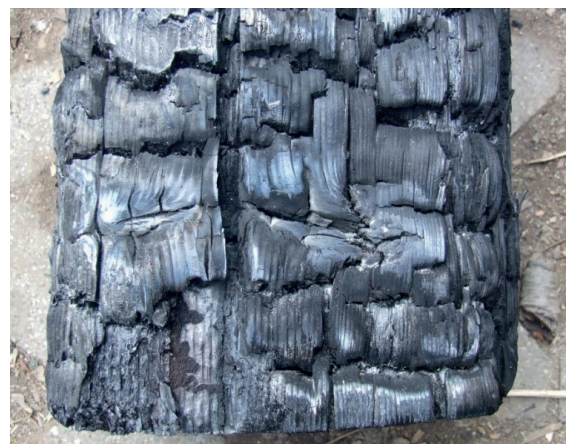
Fig. 9 Cracks on the carbonized surface (made by the authors)
