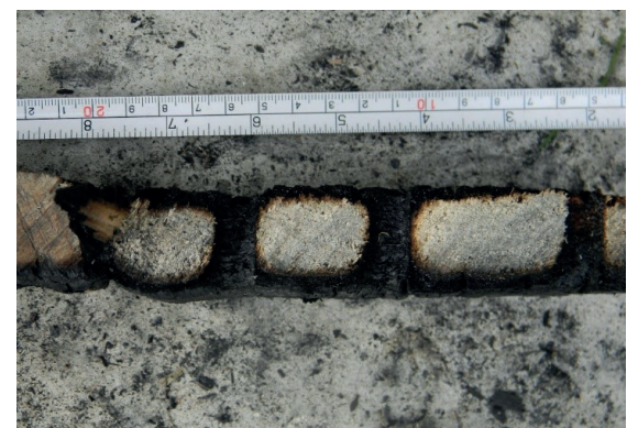
Fig. 11 Discolouration at the screws (made by the Authors)
