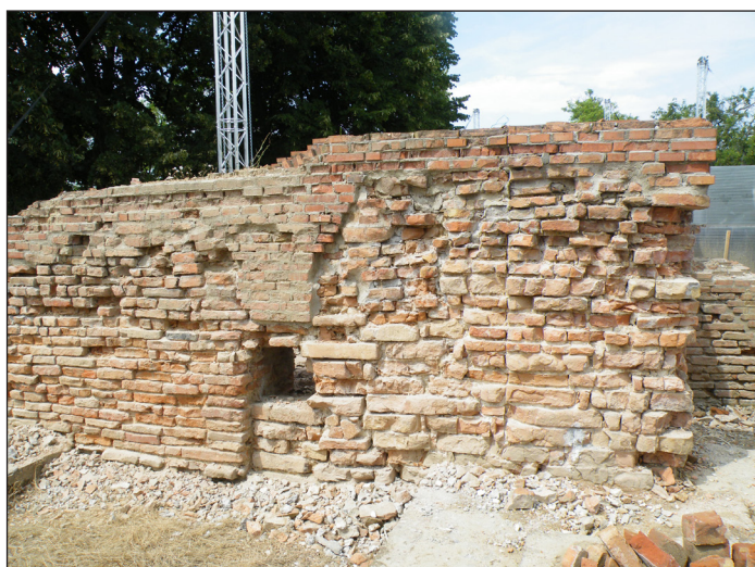
Fig. 5. The reused wall sections of the early church can be easily distinguished in the picture taken during the renovation of the monument
