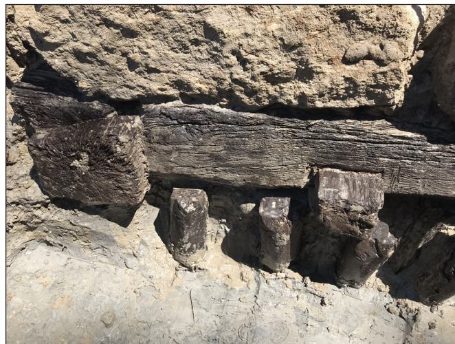
Fig. 9. Detail of the jointed beam structure and row of piles on the northern side of the bridge aperture (photograph by Barbara Hajdu)
