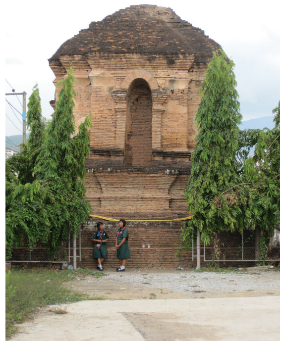
Fig. 3: Tilted buildings citywide
