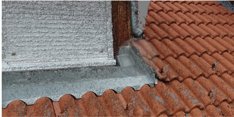
Fig. 4. Point cloud detail of the surveyed roof from video exported images (Source: Olivér Rák)
