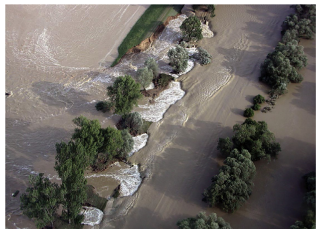
Fig. 4. Destruction of the right bank dike in 2010 (Photo: Kolesárová, SWME)
