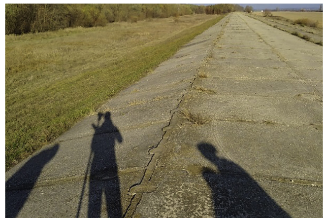
Fig. 6. Photo of 250 m long solid lateral spillway in the left-side protection dike (Photo: Soltész)
