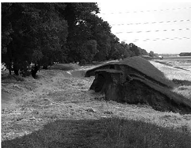
Fig. 2. Damaged left side protection dike on the Ondava River in 2004 (Photo: Kiss, SWME)
