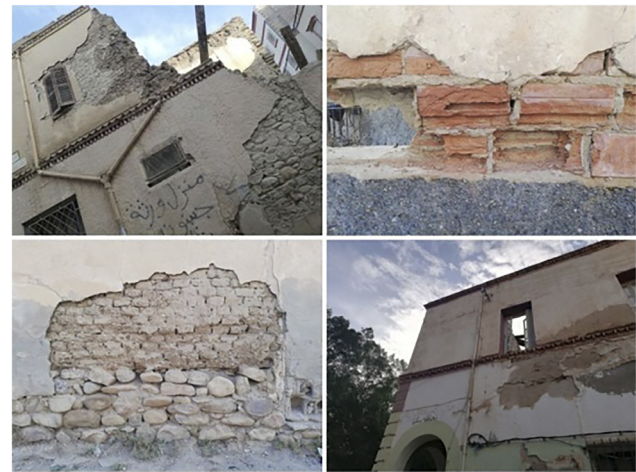
Fig. 5. Major problems affecting the construction materials (Source: Author)
