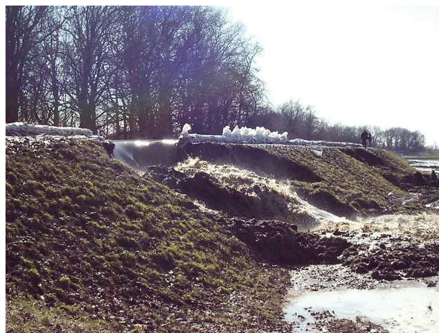
Figure 6 | The beginning of the dike failure in 2001 at Tarpa Source: ABKSZ
