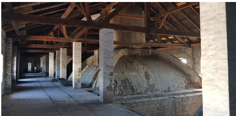
Figure 16. Brewery Dreher, oast houses, roof structure. Budapest, Kőbánya, from 1875. (Photo: Martin Pilsitz)
