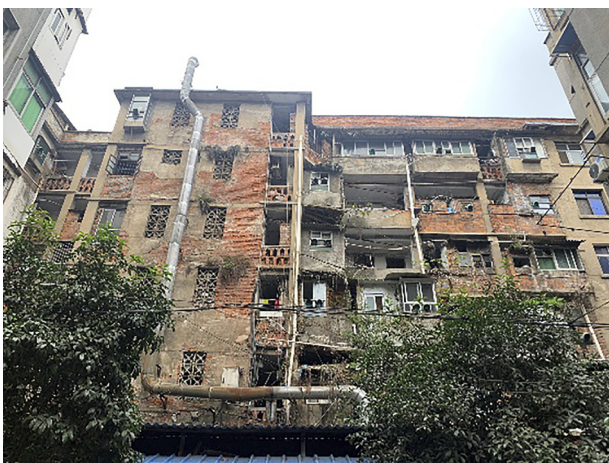
Fig. 6. Façades damaged of residential buildings of Feng Ye Shan community (Photographed by Pan Hao Wei)
