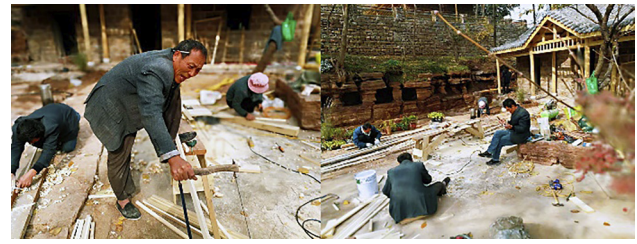
Fig. 3. Liang Wang Bie Yuan construction process by traditional house building techniques (Source: Photographed by H. Cao and E. Q. Zhang)
