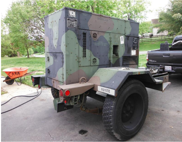
Figure 3. US MEP–805A 3 tons towed military generator driven by a John Deere 4 strokes diesel engine. Max output is 30 kW AC. It has EMP proof capability and quiet working method for tactical missions. [18]
