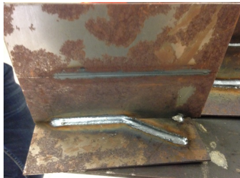
Fig. 2 Misalignment of the weld without arc sensor
