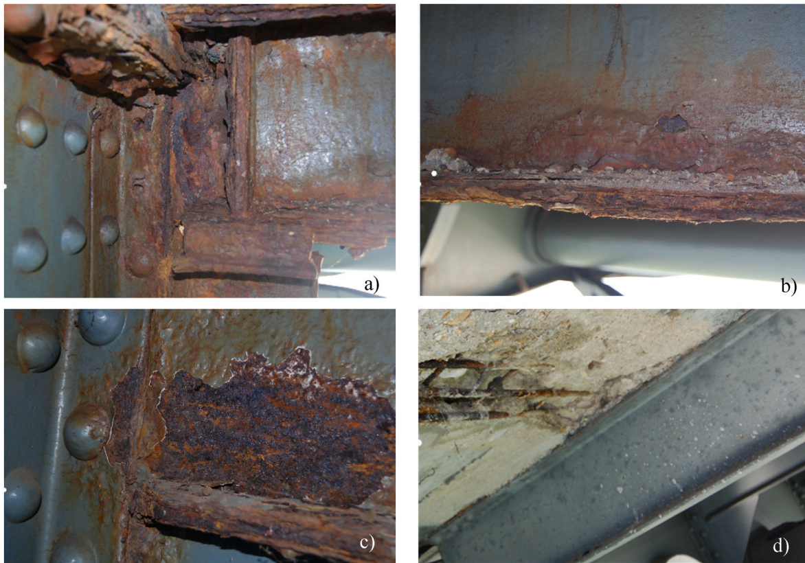
Fig. 9. Corrosion state of a) outer longitudinal stringer near the expansion joint, b) lower flange of outer longitudinal stringer, c) smaller areas with local corrosion defects and d) inner longitudinal stringers (Source: Provox Híd Ltd.).
