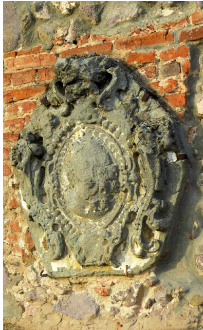
46. The damaged Rákóczi coat of arms on the wall of Mukachevo Castle
