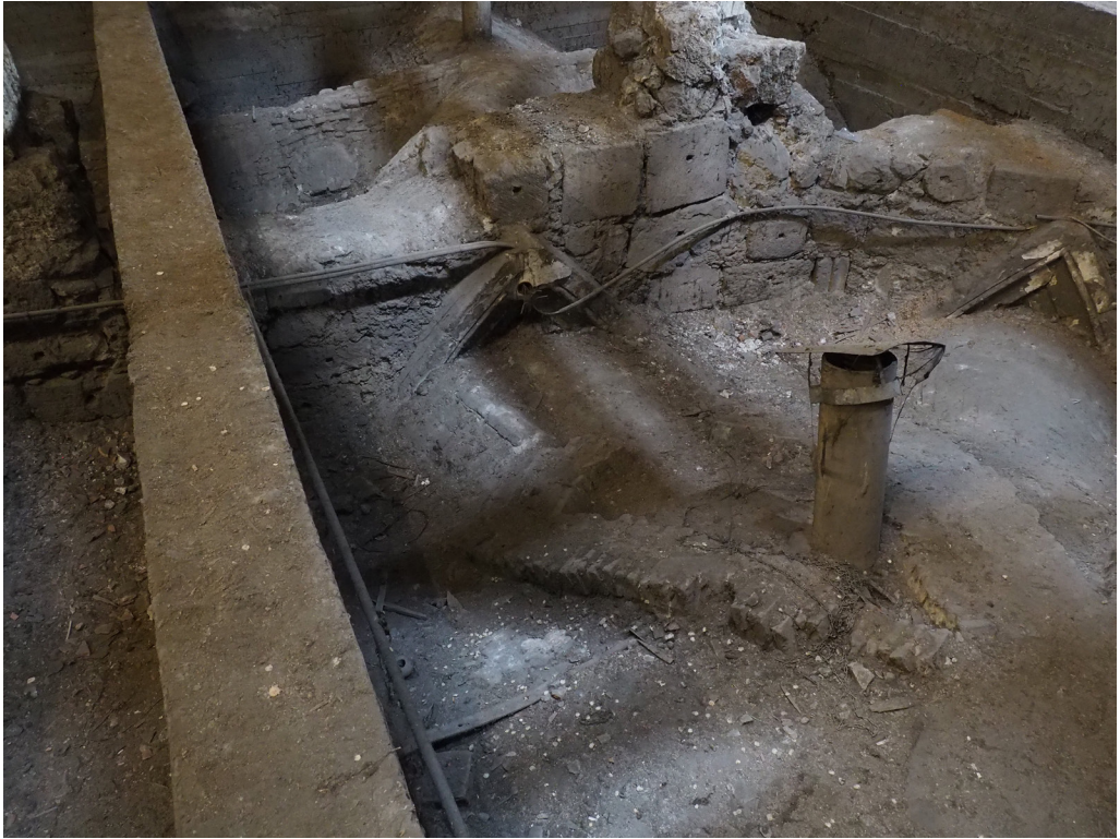
Figure 6. The remains of the wall arches above the present polygonal vault (Photo: the Authors)
