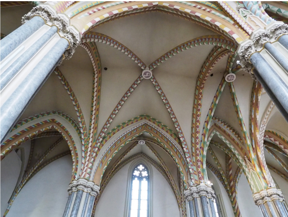
Figure 1. Detail of the cross-vault system in the apse of the Inner City Parish Church of Budapest (Photo: the Authors)
