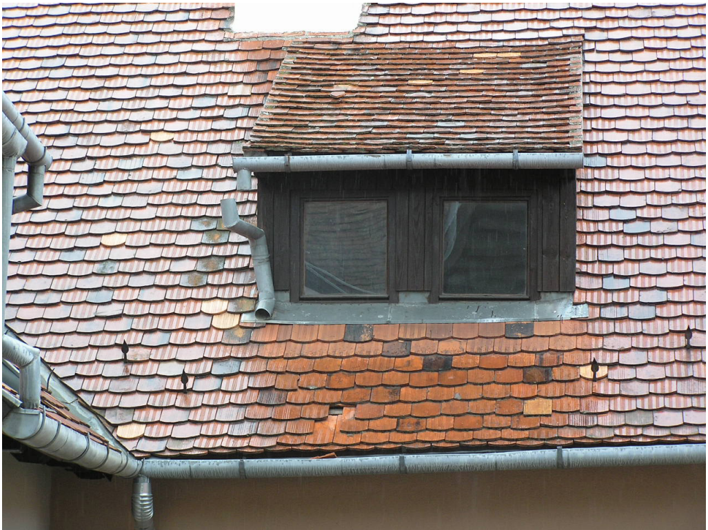
Figure 11. Tiles and gutters that have slipped due to lack of maintenance. Small jobs not performed can lead to much bigger damages (Photo: the author)
