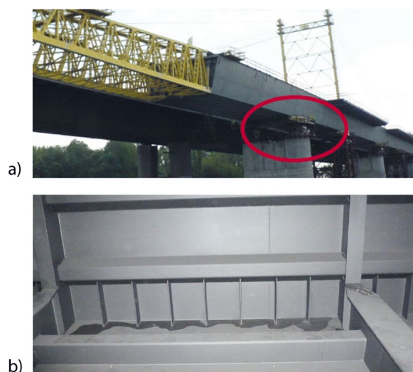
Fig. 1 Typical layout of the launched box section bridge a) launching phase and b) internal stiffeners to avoid patch loading failure
