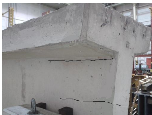
Fig. 1 Spalling crack in the end of the beam
