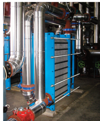
Figure 7. Heat changers before the heating circulation
