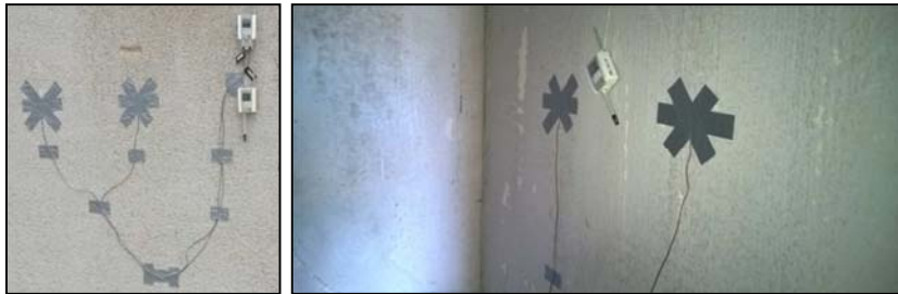
Fig. 11. Saveris data collectors on the southern wall outside (left) and inside (right) measuring air temperature, surface temperature and relative humidity
