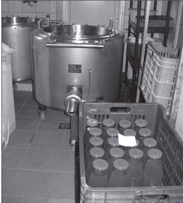
Figure 6. “Taste House” is a processing plant with state-of-the-art technology. Hernádszentandrás, Hungary, 2016. (Photo by Anikó Báti)
