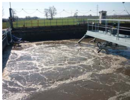
Fig. 4. Aeration tank of WWTP Vráble
