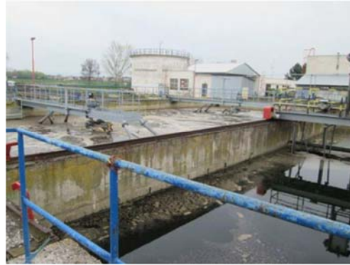
Fig. 6. Sedimental tank of WWTP Vráble
