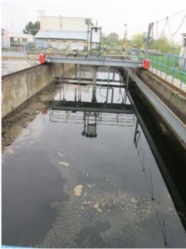
Fig. 5. Sedimental tank of WWTP Vráble
