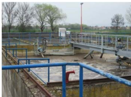
Fig. 3. Aeration tank of WWTP Vráble
