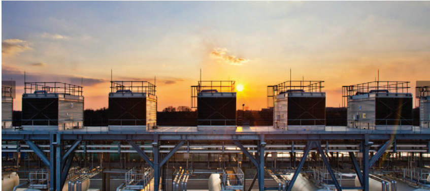
3. Figure: Water tanks and cooling towers of Google in Belgium 17
