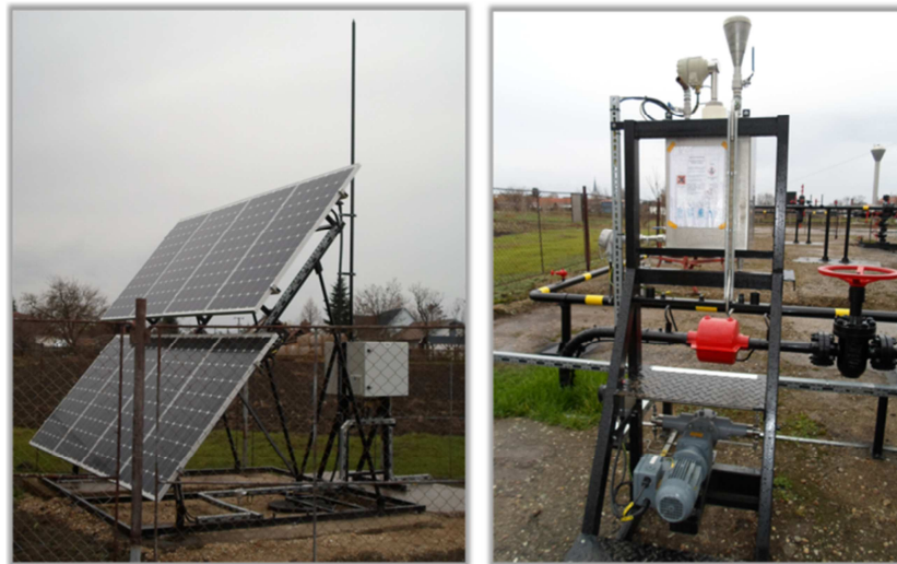
Fig. 3. Pump system (source: Research Institute of Applied Earth Sciences, University of Miskolc)
