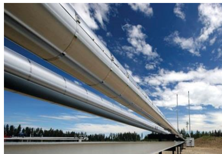
Fig. 1. An above-ground pipeline
