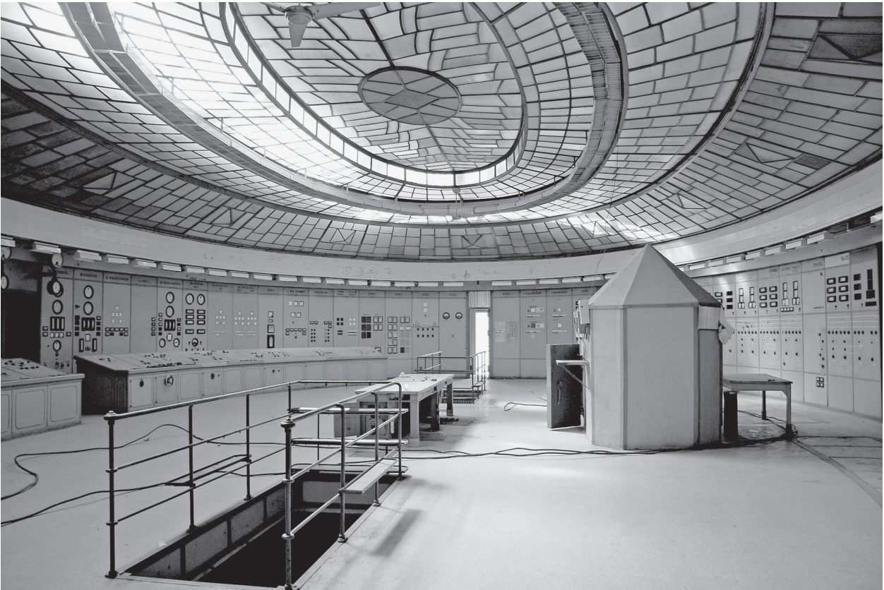
Fig. 18. The control room of Kelenföld Power Station (photo: Galacánu Efstatia, 2008)
