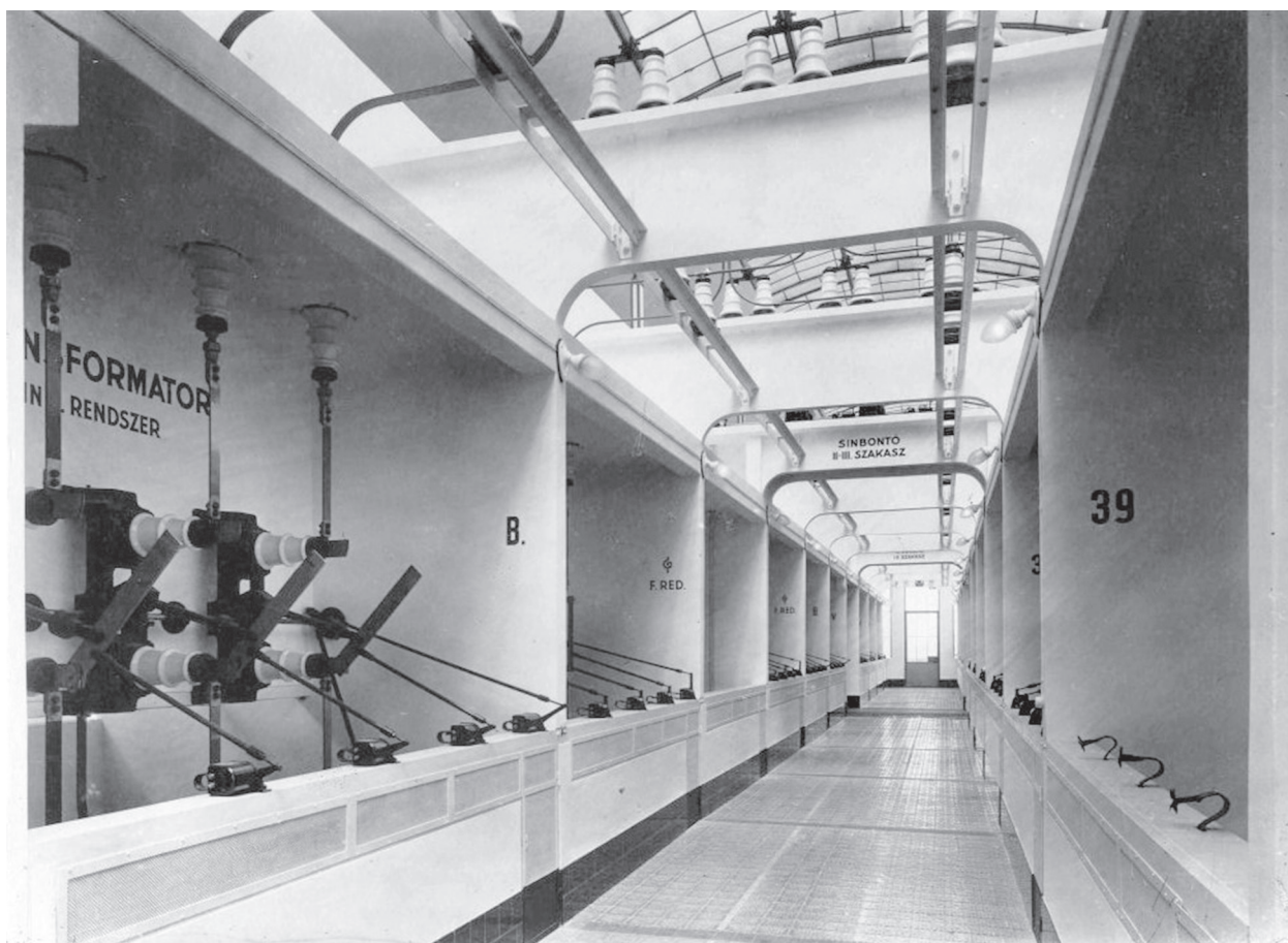
Fig. 16. The basement of Kelenföld Power Station, architects: Kálmán Reichl and Virgil Bierbauer, 1913/1927–1933 (photo: Ernő Bánó, 1933; IPM FLT 24468.4)
