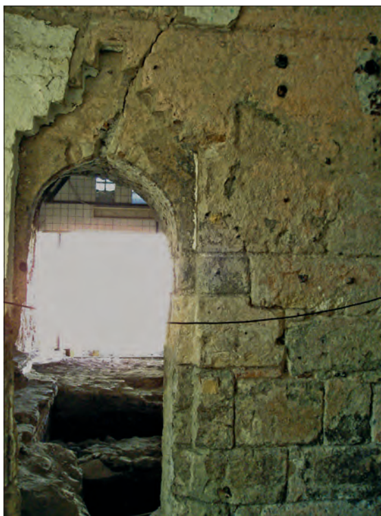
Figure 81. Stepped ornamentation of the door between the warm rooms at the Rudas Baths during excavation
