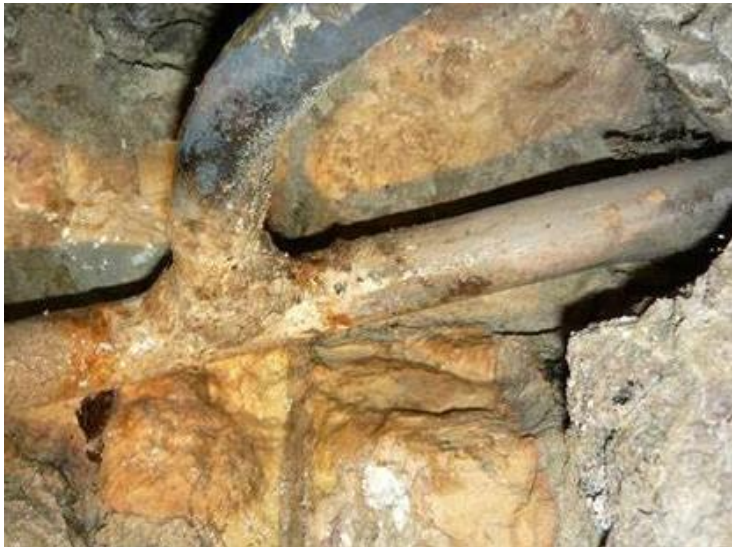
Photo 2. Exploration of worn corroded pipes in concrete-stone foundation
