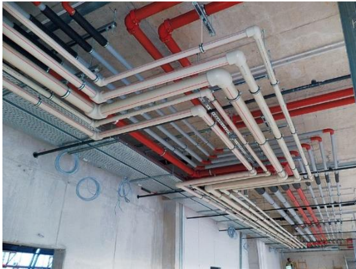
Photos 3-4. Plastic pipelines and an optional placement. Source: 19
