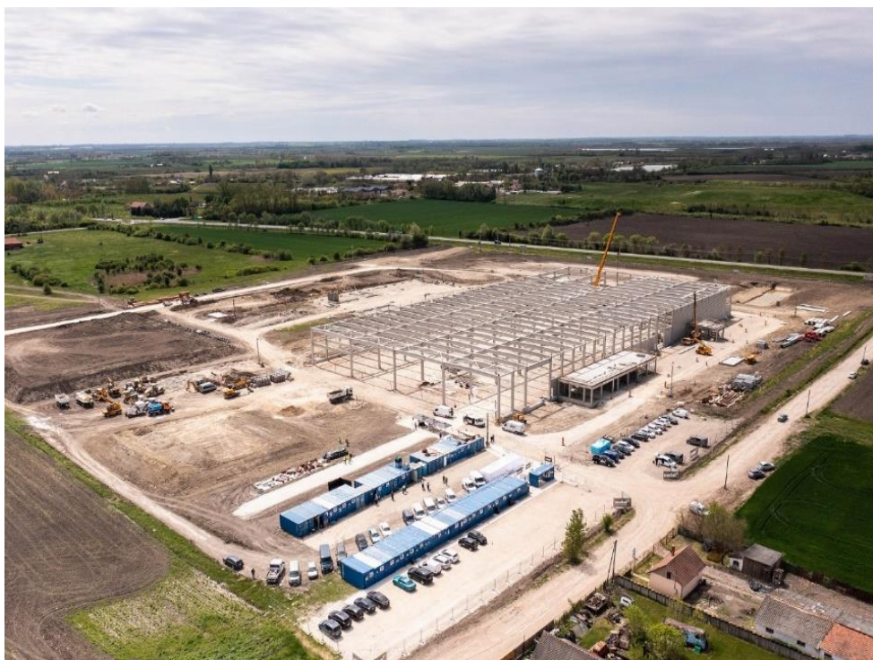
Figure 4: The construction site of Airbus Helicopters Hungary plant at Gyula is being overflowed by a Hungarian Defence Forces H145M helicopter
