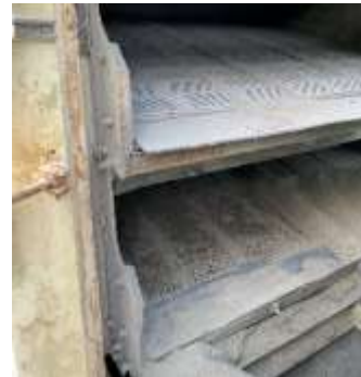
Figure 11. Clogging of a lower screen deck.
