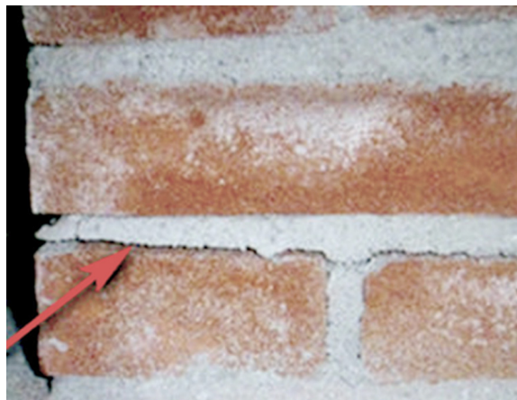
Figure 1. Opening crack between mortar and brick
