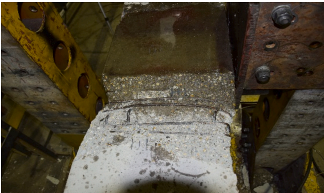
Fig. 19. Concrete flange failure (B2) – view from above.
