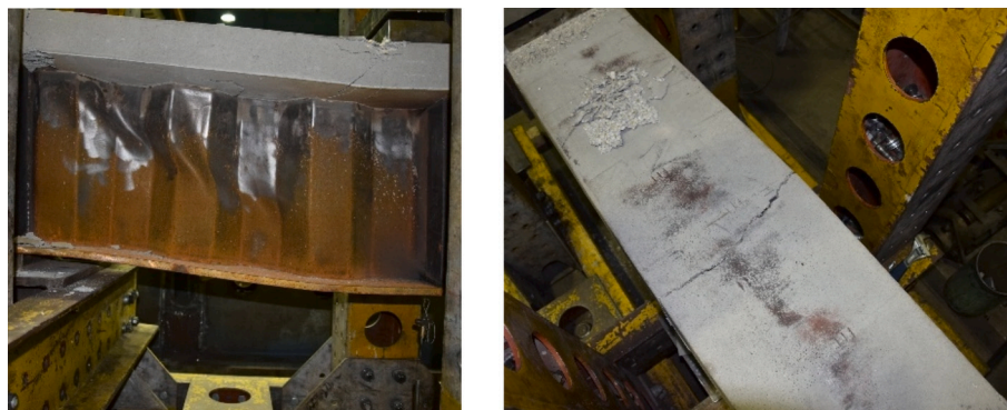
Fig. 17. Web buckling of B1/3; Concrete cracks above the support (close to the load).
