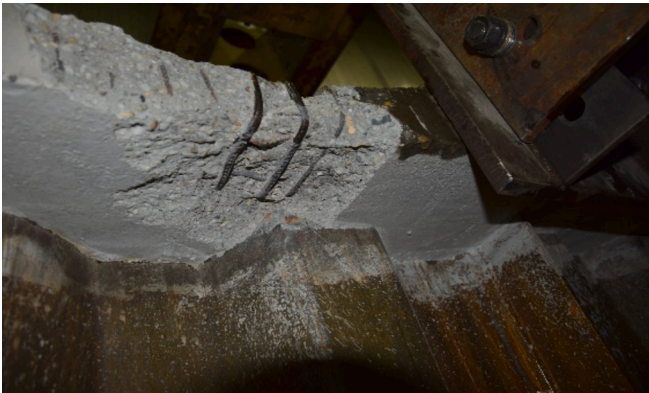
Fig. 20. Concrete flange failure (B2) – view from below.
