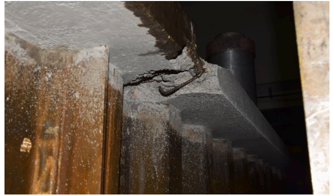
Fig. 21. Damage on the upper concrete flange (B2).
