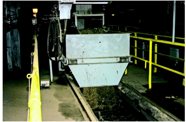
Figure 7. The system of boiler feeding with the coal and biomass mixture
