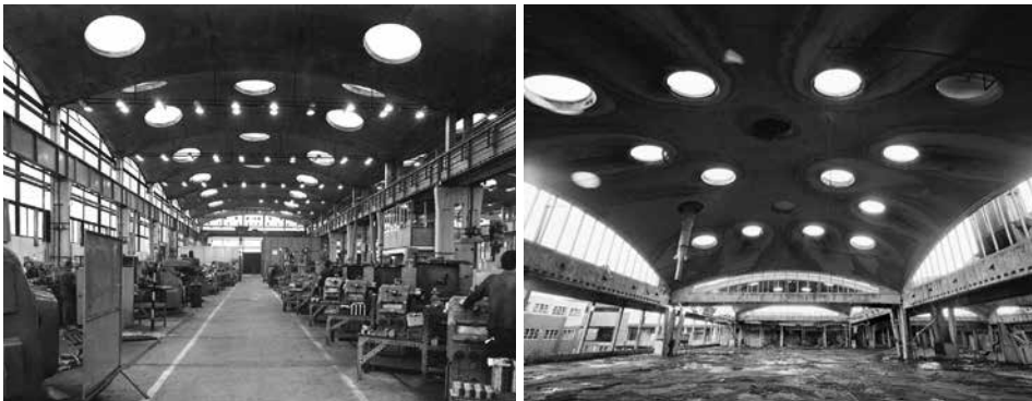
Figure 15. Csepel factory hall (1967) (l), archive and Brynmawr Rubber Factory (r), prior to its demolition showing signs of leaking around the skylights
